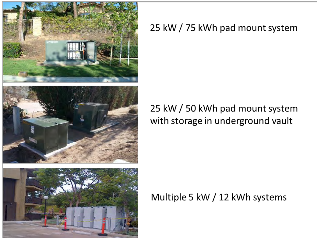
Figure 14 – Example ESS Installations
