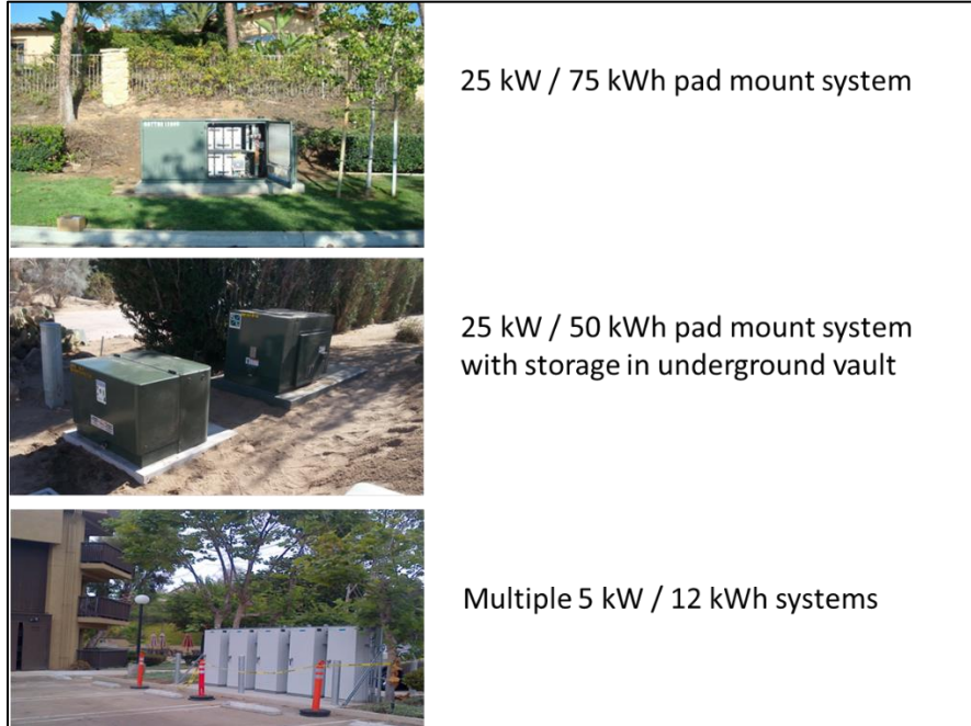
Figure II-L – Example ESS Installations
